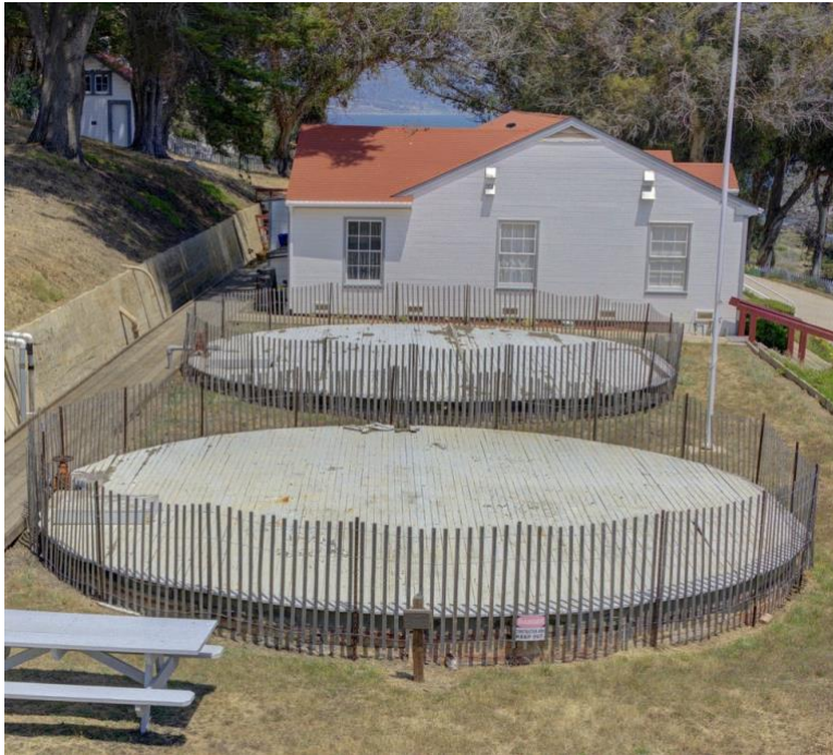
Point San Luis cisterns, urgently in need of restoration. Photo courtesy of Bob Mihelic.
