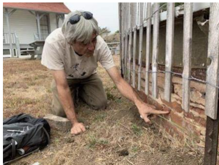
Dan Mosier, California brick expert, examining the cistern bricks in August 2019. His examination confirmed the bricks came from the Ah Louis brickyard in San Luis Obispo. Photo courtesy of the Point San Luis Light Station archives.
